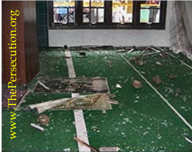
An inside view of the damaged Mosque
